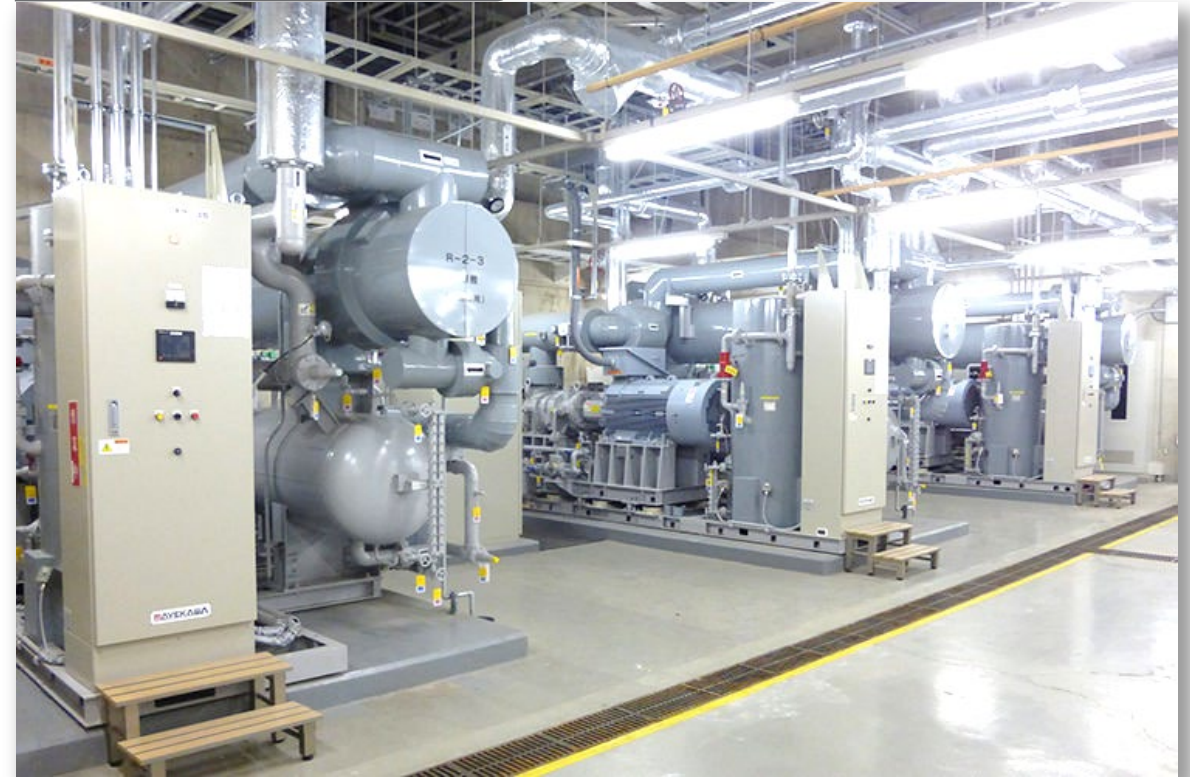
Energy Transfer Plant
